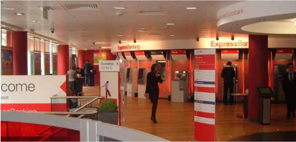
HSBC, QUEEN VICTORIA STREET, LONDON £9m fit out of the biggest bank in the UK, including new service lifts, staircases, façade alterations and CAT A fit out works.
